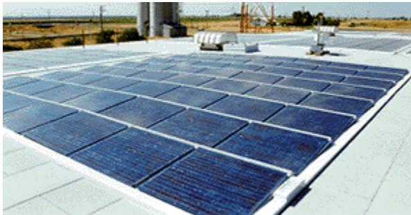
PV tiles on the roof of a commercial building (PowerLight Corporation)
